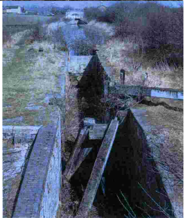
The remains of the second lock from Norbury on the Newport Branch in the mid 1960s.
